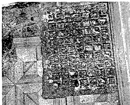
Healthy Homes unit in Cambridge: Debris-Filled Floor Vent
