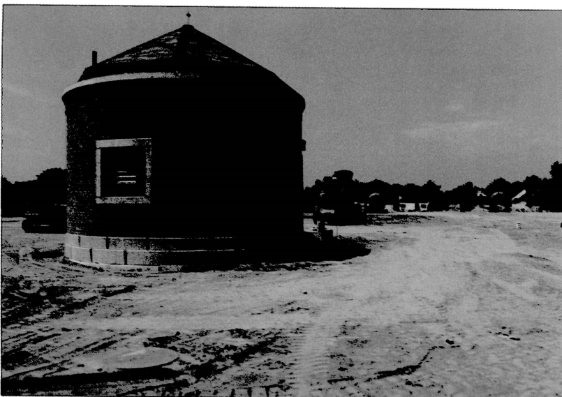
July 1991 — Newly covered tanks in both basins backfilled and ready for use.
